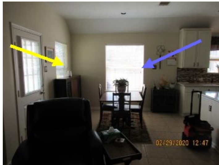
These windows are hard to operate. The blue arrow points to a hard to open and close/lock one. The yellow arrow points to one that I could get open but could not get it down far enough to close and lock.
