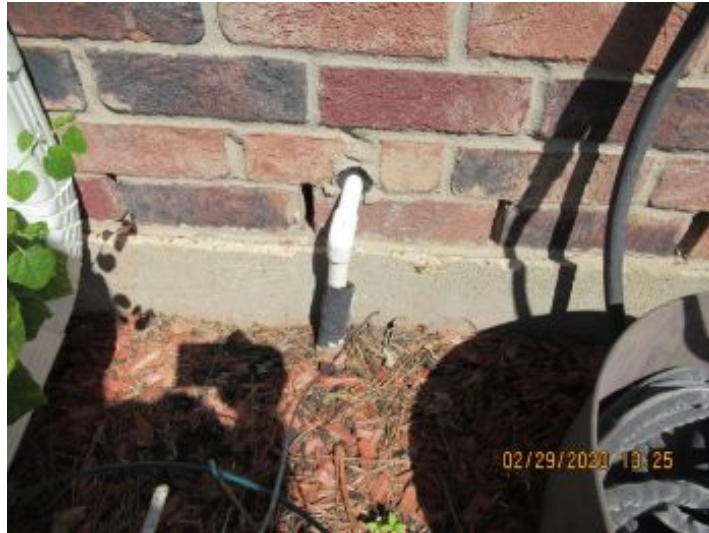
This piping is missing insulation.
