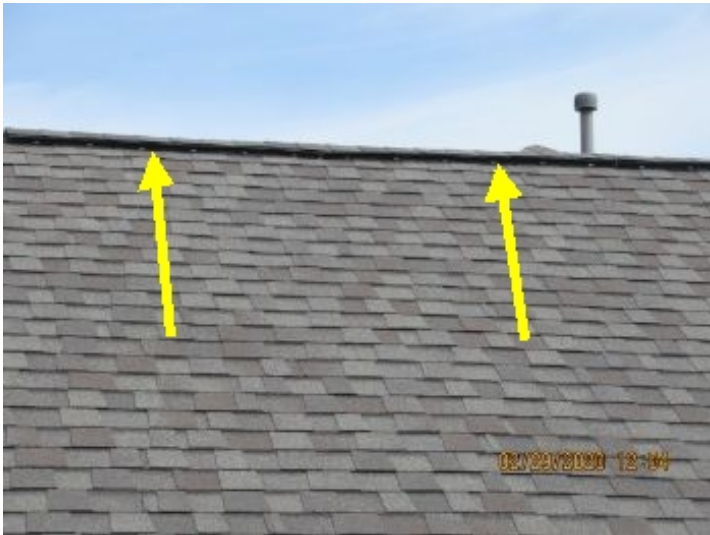
The ridge vents are part of the attic ventilation system and allow the hottest air to escape.
