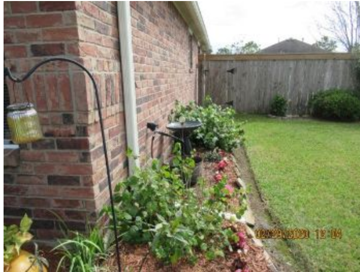
Grading and drainage appears to function as intended at the time of the inspection but this wall also has foliage growing against it that should be trimmed.
