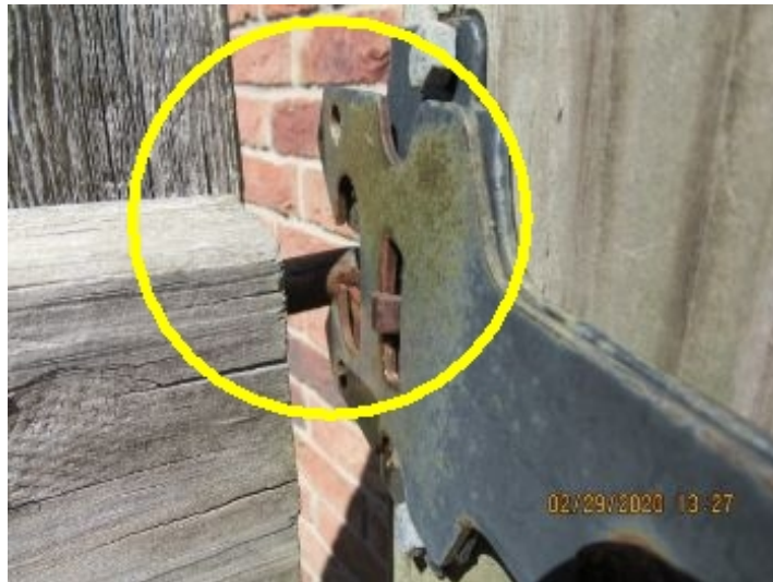
The latch on the gate is hard to lock and should be fixed or replaced.
