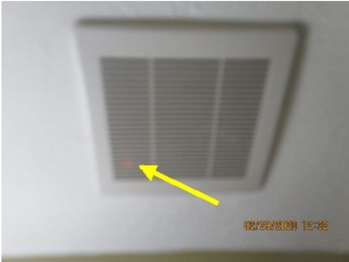
This is the humidity controlled exhaust fan. You can see the faint orange color that shows it is running. When powered but not running, the light will be blue.
