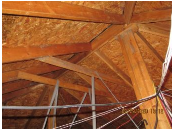
This is a good shot of some of the framing that appears to function as intended at the time of the inspection.
