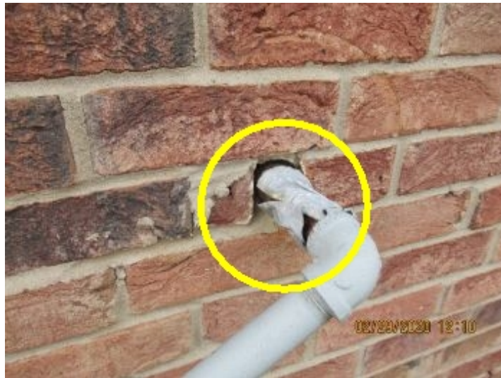
Wall opening needs to be sealed.
