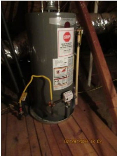
New 40 gallon Rheem water heater installed and functioning as intended at the time of the inspection.
