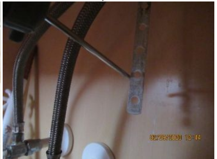
because the stopper rod is not connected below. This is a small thing that can easily be corrected.
