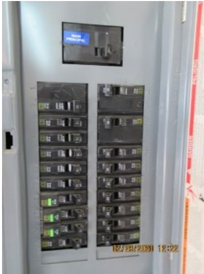
The 125 Amp electrical panel appears to function as intended at the time of the inspection.
