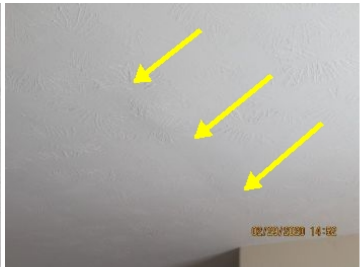
This is a belly in the ceiling between the den and the breakfast room ceiling that is also evidence of a past water leak. I was told the roof was replaced last year.
