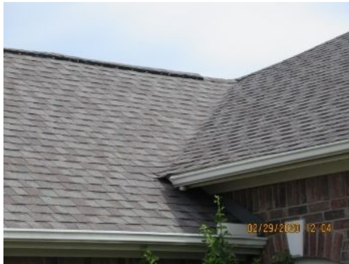
Roof is approximately one year old and appears to function as intended at the time of the inspection.
