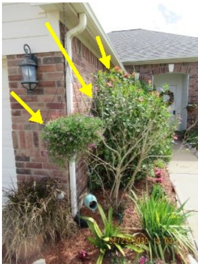
All foliage should be trimmed away from the exterior veneer 18" to allow for air circulation to allow moisture evaporation.
