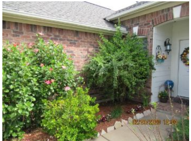
Another view of foliage that needs to be trimmed to allow air circulation between the bushes and the brick.
