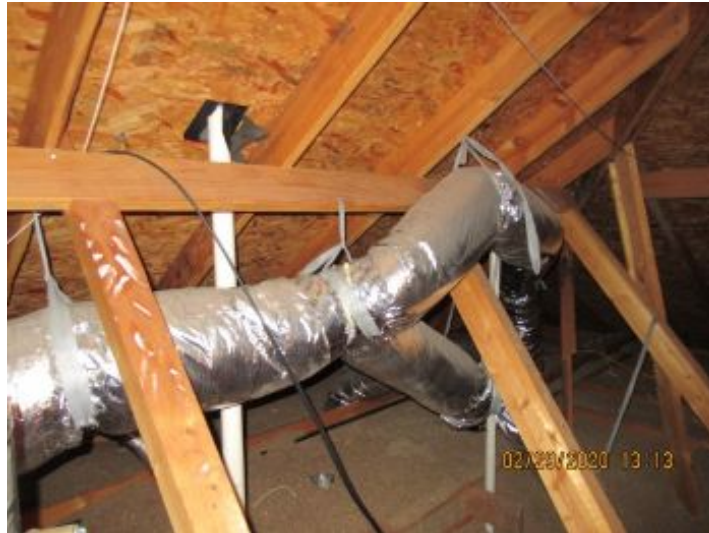
Ductwork is supported as suggested and appears to function as intended at the time of the inspection.
