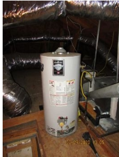
Old Bradford-White water heater that the plumbers did not remove but should have.
