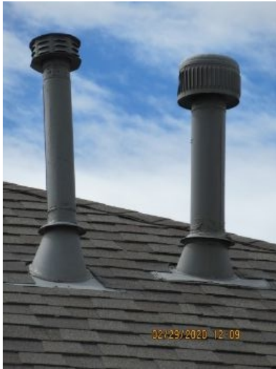
The roof vents appear to be functioning as intended at the time of the inspection.
