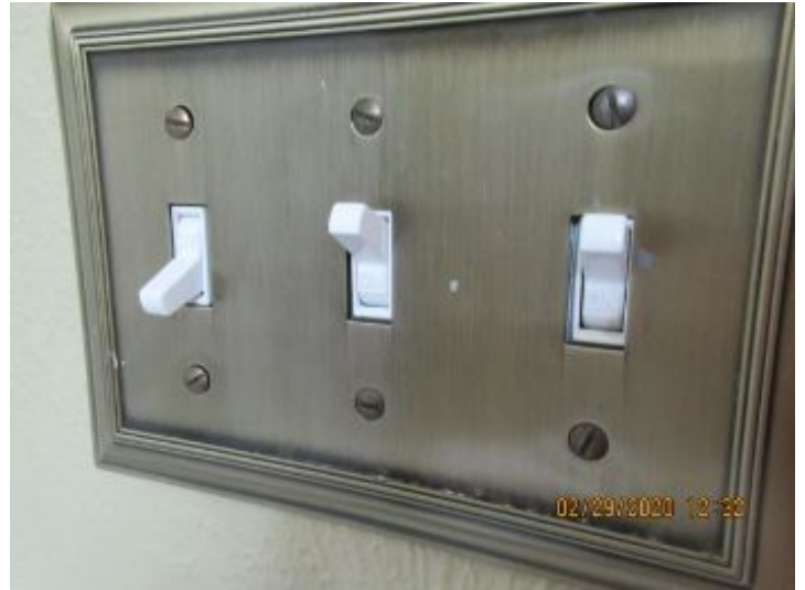
The middle switch of the hallway bathroom gives power to a humidity controlled exhaust fan.
