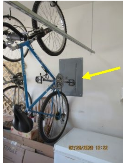
Had to move bike to check out the electrical panel.
