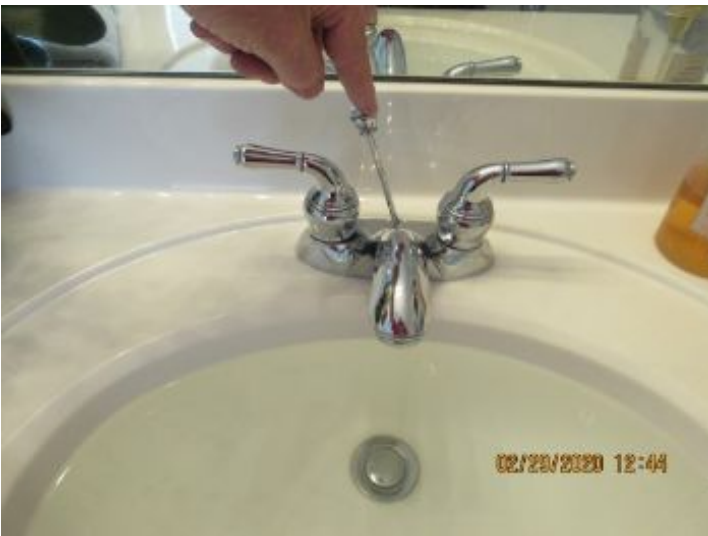
In the master bathroom, the right sink's stopper is not working...
