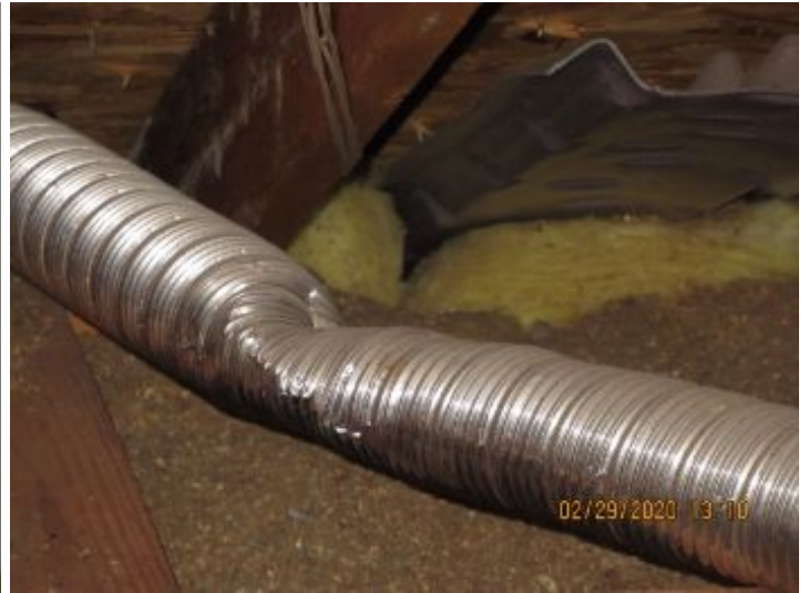
This ventilation piping is bent and should be repaired and/or replaced.
