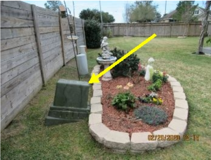
This is the underground feed for the electrical power for the house.
