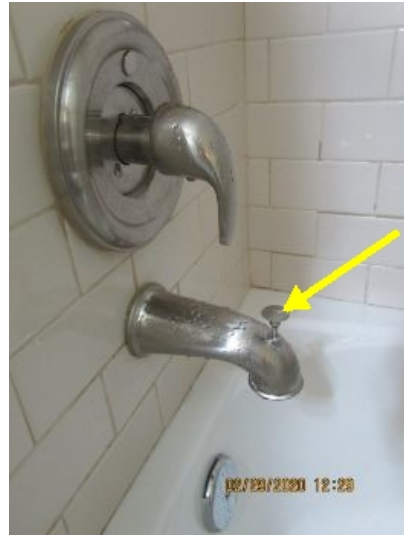
In the hallway bath, this shower/tub lever is too hard to operate. Downward pressure could possibly bend the water supply pipe and needs to be fixed. Suggest calling a professional plumber to fix.
