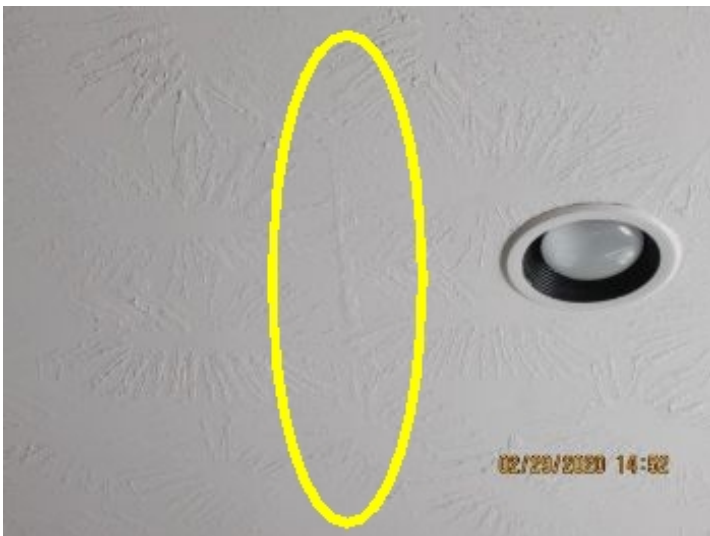
This is a small crease in the breakfast room ceiling that is typical of a past water leak or sheetrock movement.
