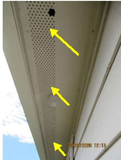
These holes in the soffit are also part of the attic ventilation system and allow the 10 degree cooler air to enter the attic as the hot air rises.
